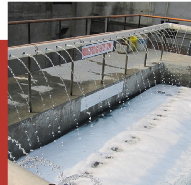
Effluent Treatment Plant
