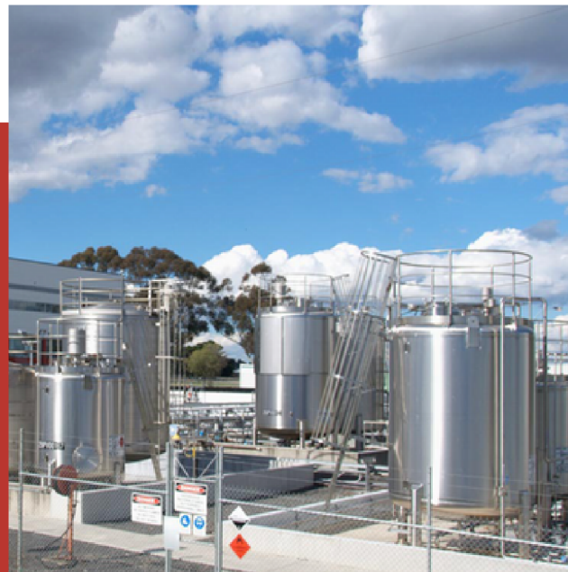
Tank Farm Installation
