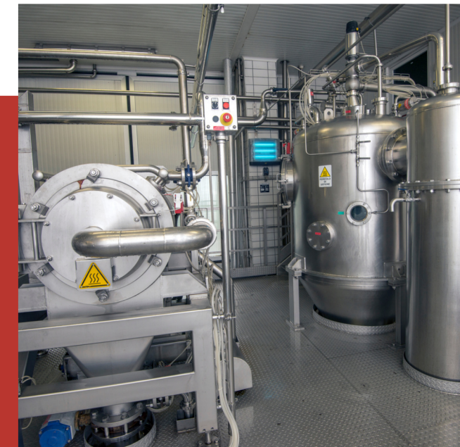
Water Purification System
